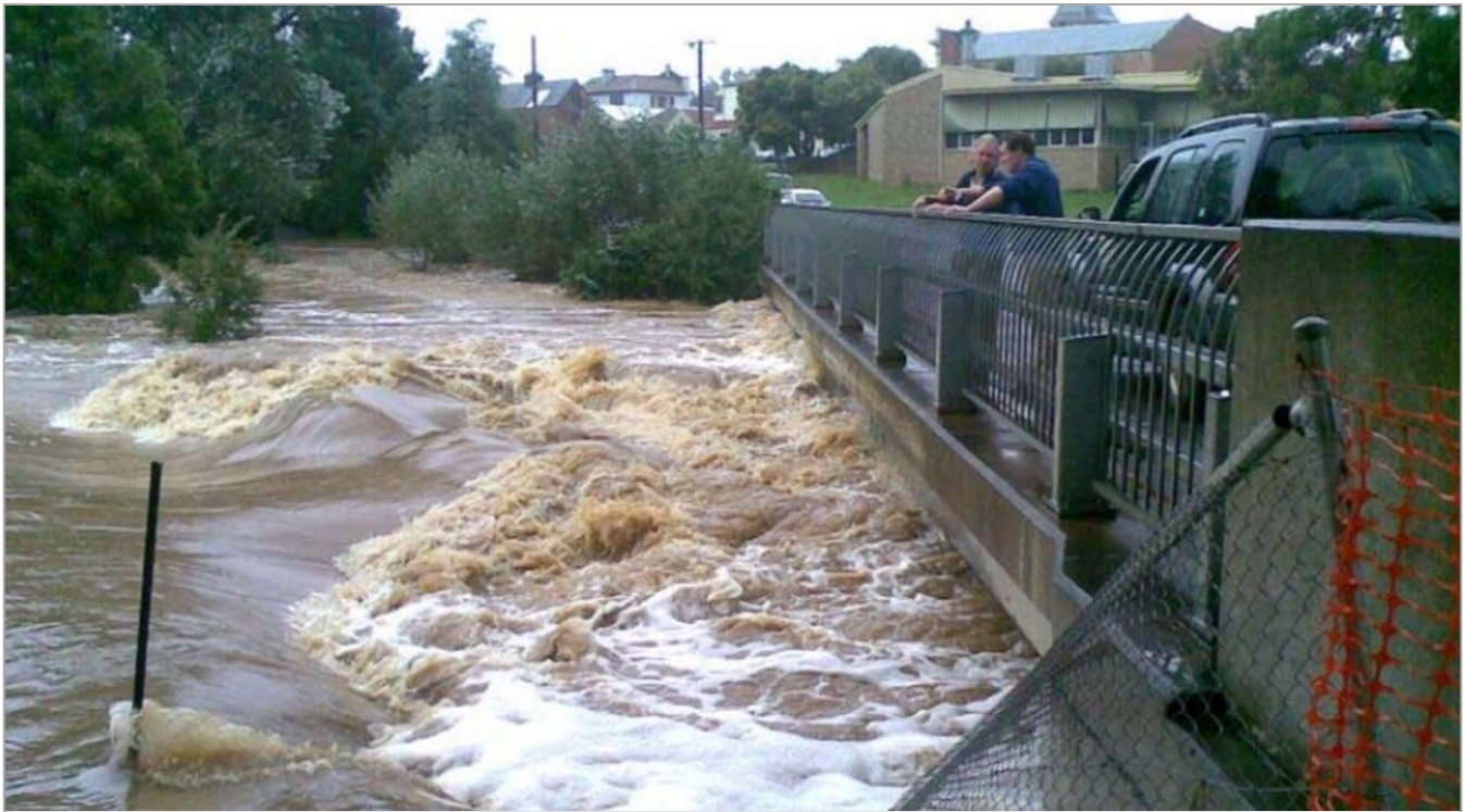
Water Street Bridge impacted by flooding during the January 2011 flood event.
