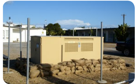
Sandbagged substation, June 2007 flood
