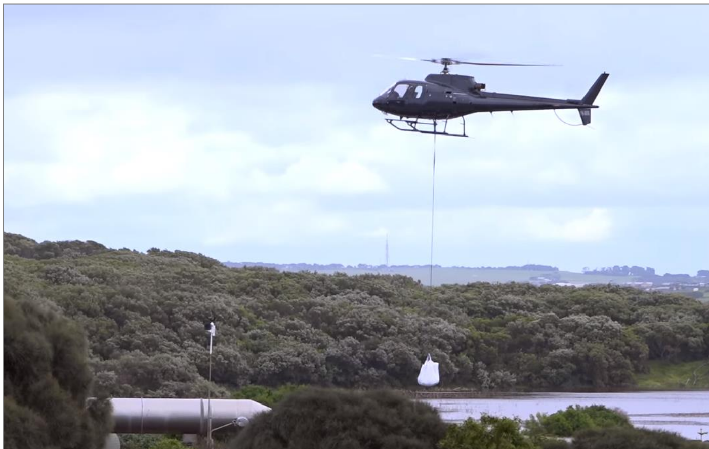
Figure 29. A helicopter dropped large sandbags to reconstruct the collapsed section of the Midfield Meat Rendering Plant levee.
