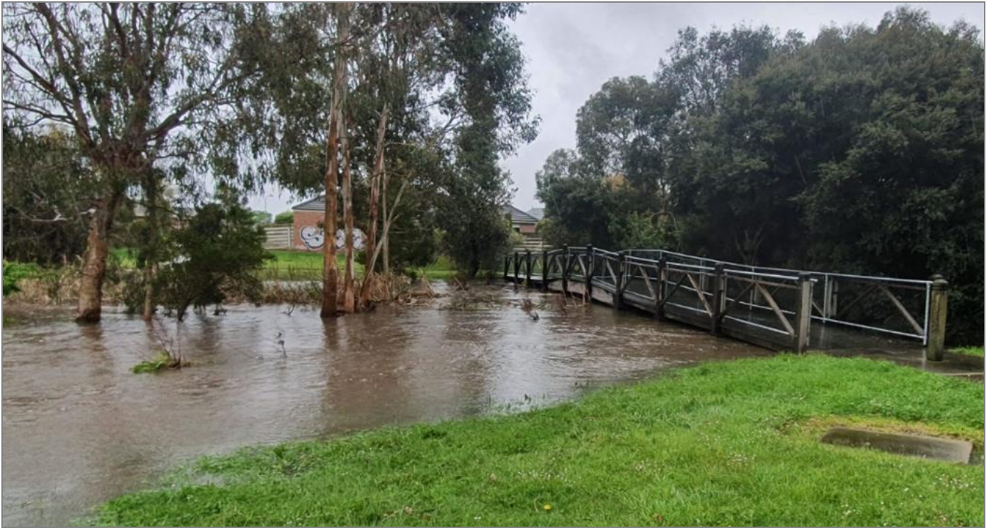
Figure 5. Flooding impacted the Russell Creek footbridge upstream of Mortlake Road during the October 2020 event.
